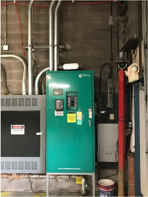
Figure EP6 - ATS and main distribution panel
