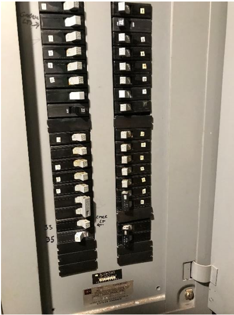
Figure EP9 - Example of existing panelboard
