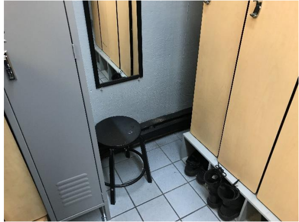
Figure 7 - Baseboard Heater located in Lower Level Men's Locker Room
