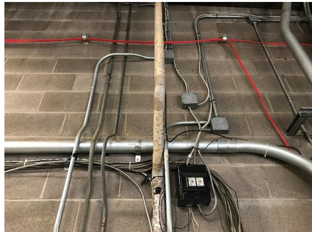
Figure EP16 - Example of improperly installed cables
