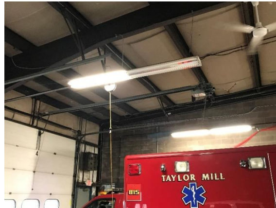
Figure EL4 - Apparatus Bay Lighting
