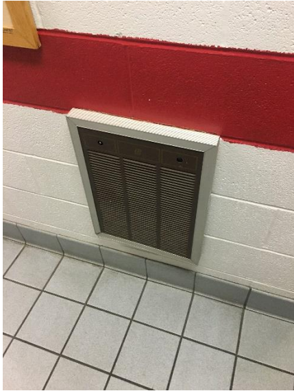
Figure 6 - Electric Wall Heater located on Lower Level
