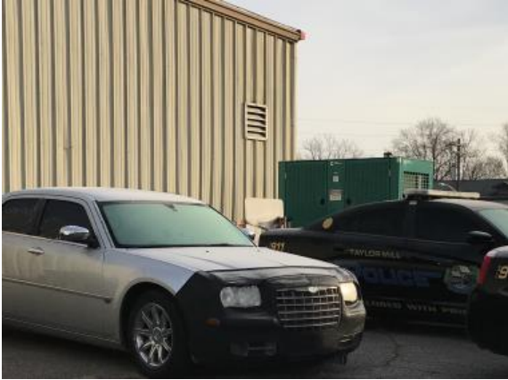
Figure EP5 - Diesel generator set behind bay building
