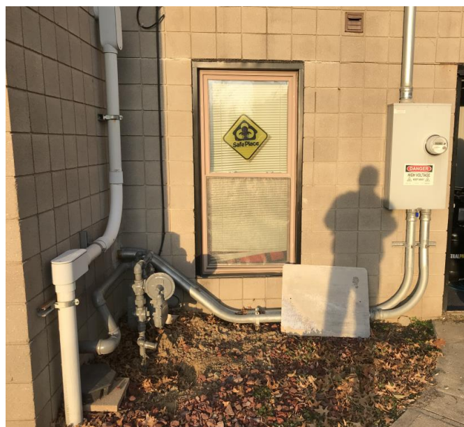
Figure EP4 - Electric utility service
