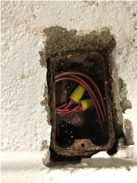
Figure EP1 - Example of aging/water damage
