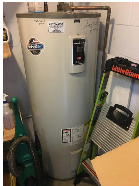
Figure 9 - Water Heater located in Lower Level Janitor Closet
