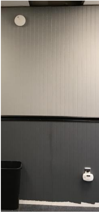
Figure FA1 - Smoke alarm unit (high) & CO alarm unit (low)
