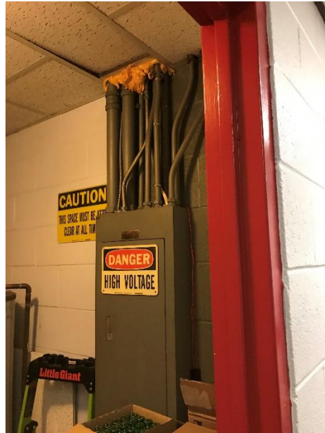
Figure EP2 - Example of trying to mitigate water damage
