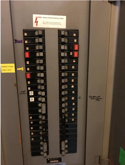
Figure EP7 - Example of existing panelboard
