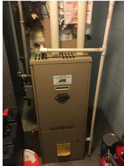
Figure 3 - Split-System AHU located on Lower Level
