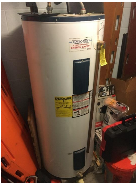
Figure 8 - Water Heater located in Lower Level Furnace Rm.
