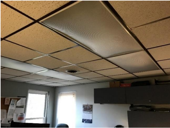
Figure EL1 - Typical Office/Living Area Lighting
