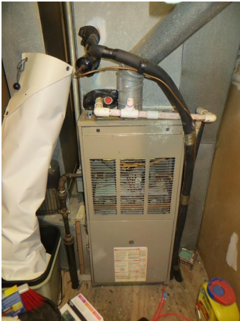
Figure 2 - Split-System AHU located on Upper Level
