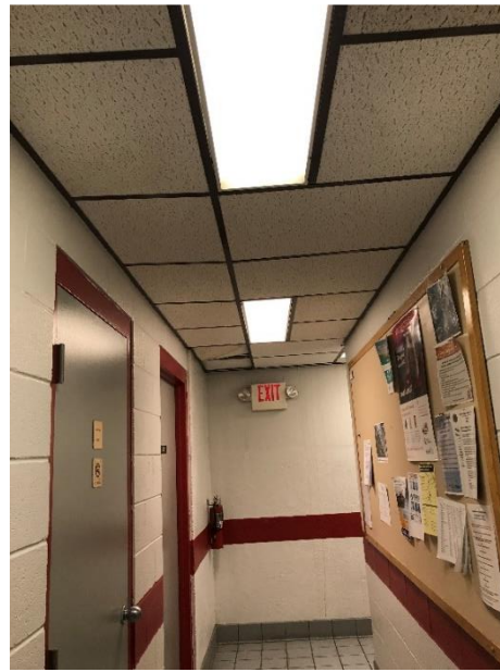
Figure EL2 - Typical Office/Living Area Lighting
