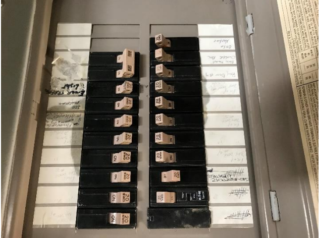
Figure EP8 - Example of existing panelboard
