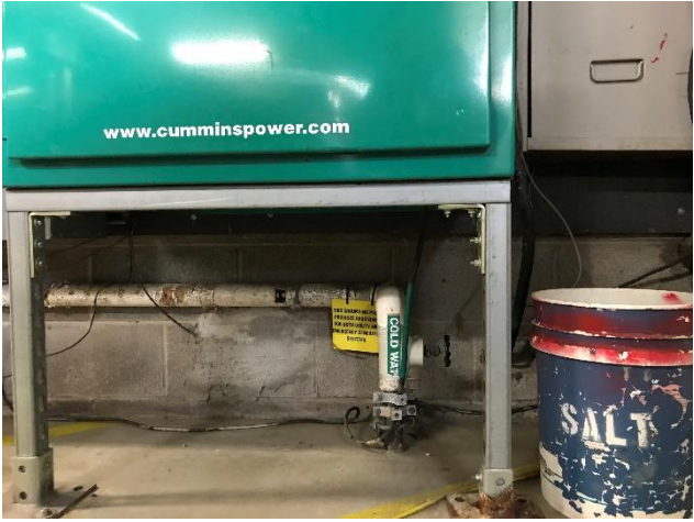
Figure EP10 - Water service entrance beneath Generator ATS
