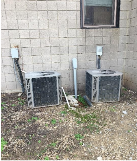
Figure 4 - Split-System AC Condensing Units
