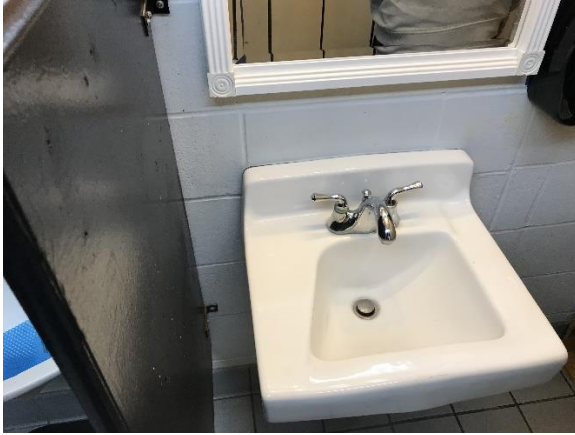
Figure 10 - Sink located in Lower Level Men's Rm. (Typical)
